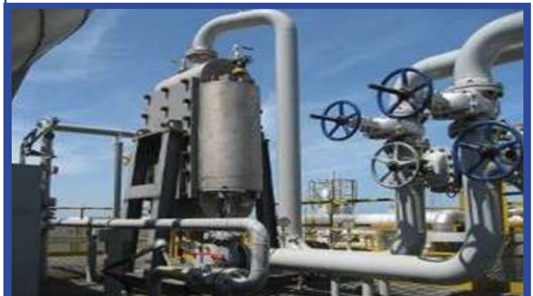
Installed Gas Processing Hybrid Heat Exchanger
